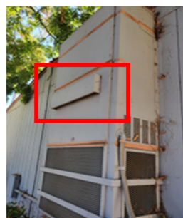
Figure 8. Outside air intake for Classroom 5, indicated by the red box.
