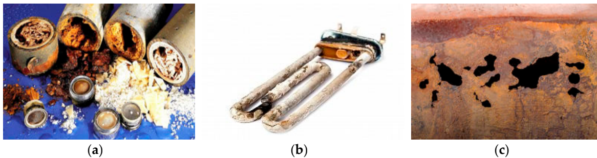
Figure 7. Effects of limestone on (a) a tube [27] and (b) the resistance of a washing machine; (c) effect of corrosion on a pipe [28].
