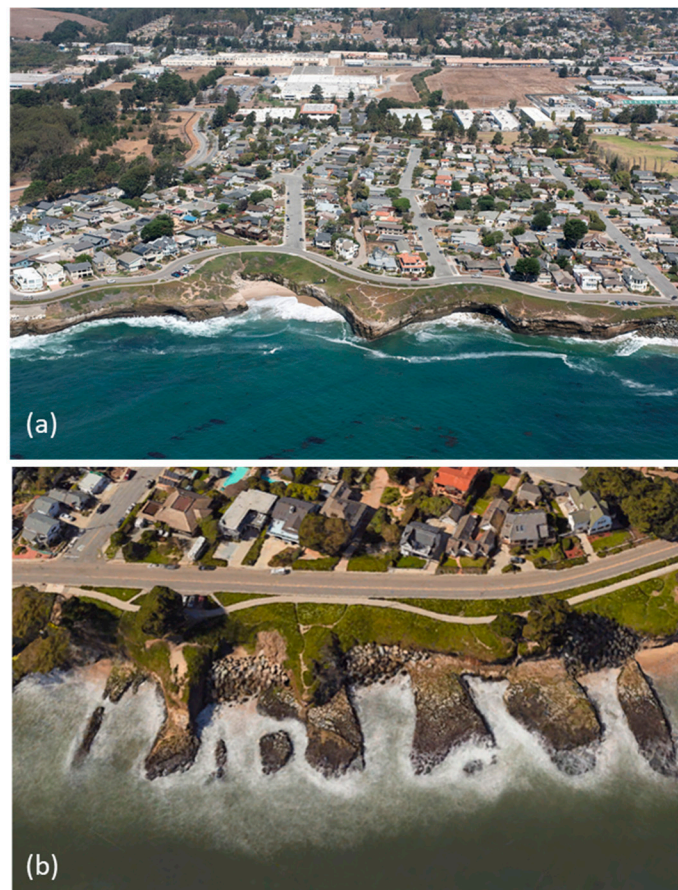
Figure 5. (a) Unprotected section of West Cliff Drive study area showing low eroding cliffs eroded into the Santa Cruz Mudstone [15], (b) oriented embayments eroded along parallel joints in the Santa Cruz Mudstone (Google Earth, 2018).
