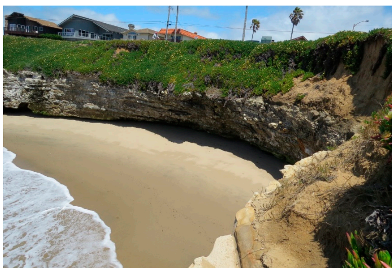
Figure 17. A section of coastal bluff consisting of the overlying weaker terrace deposits that are mostly vegetated, and the underlying Santa Cruz Mudstone that is being undercut. As in Figure 6, selecting the edge of the bluff for comparative measurements is difficult and somewhat subjective.
