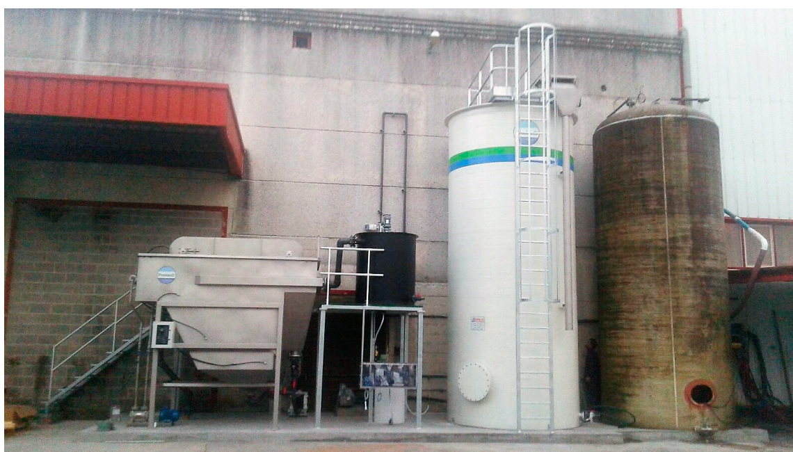
Figure 3. New pretreatment installed in February 2018 by company 3.
