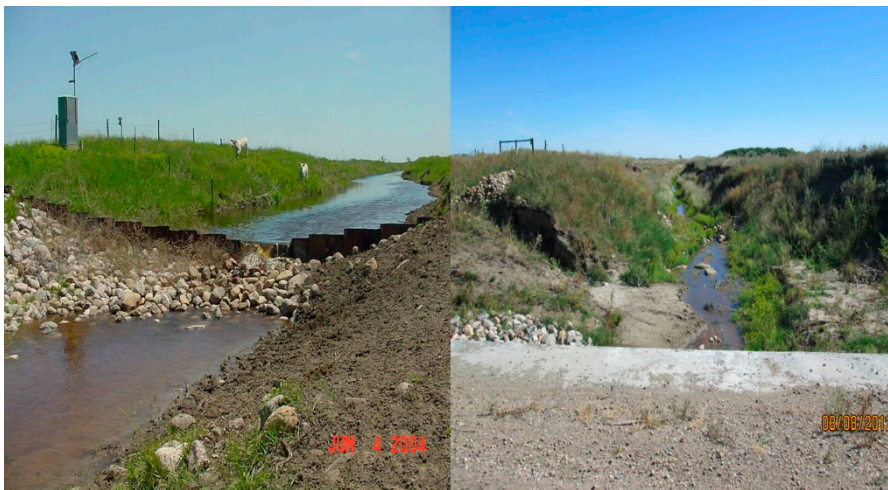
Figure 5. Rock and sheet pile weir (installed in 2001) at the Road 1212 crossing in June 2004 (photo from B. Braun, U.S. Forest Service) and at the same location in August 2012 (photo from P. Gerla).
