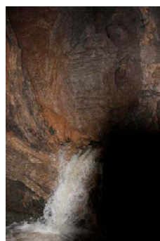
(e) Water can pour through the cavity exposed in the tunnel cross section after a short burst of rain on the surface.
