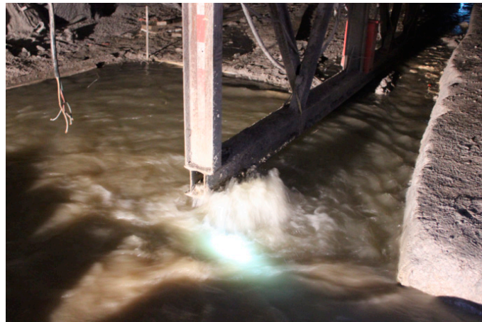
(f) Water gushing from the tunnel-floor cavity.
