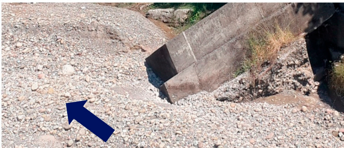
Figure 1. Failure of spur dike at the river Gaula near Haldwani, Uttarakhand in India.
