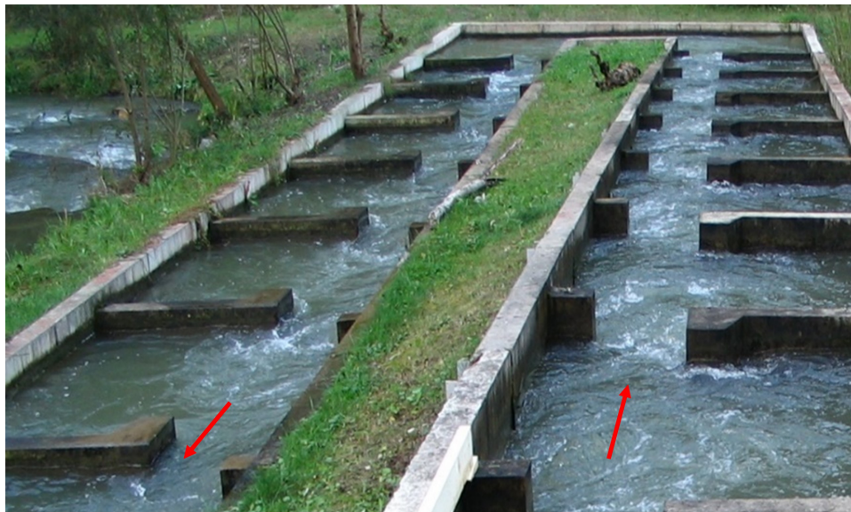
Figure 7. Prototype VSF at Arto-Blanca HPP during field measurements.
