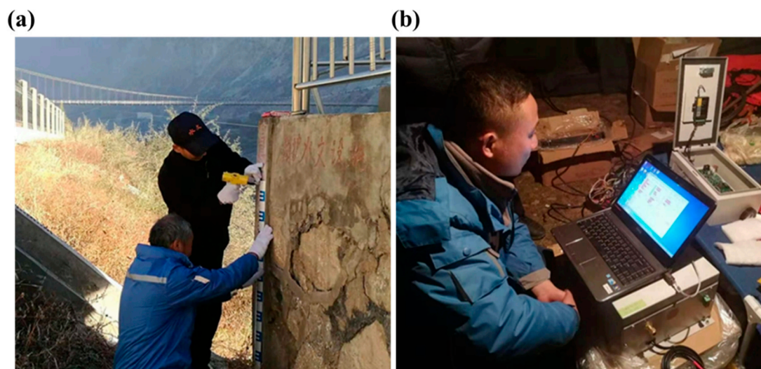
Figure 5. Hydrological monitoring in the downstream of Baige landslide. (a) Installation of water level ruler; (b) testing hydrological monitoring equipment.
