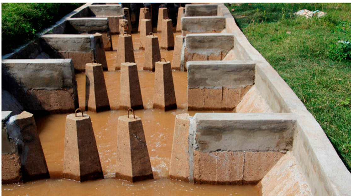
Figure 2. The cone fishway at Pak Peung village. The fishway had 1.0 m-high concrete cone baffles set up in two alternating arrangements—one with three full slots and the other with two full slots and two half slots (source: Lee Baumgartner). Each set of baffles was separated by a 2 m long by 3 m wide pool, which had a depth ranging from 0.6 to 1.5 m depending on the flow through the fishway. The sloping channel walls, low depth and low energy pools also made for safe human access and egress, which was a site-specific requirement in the remote village where children regularly interact with the fishway.
