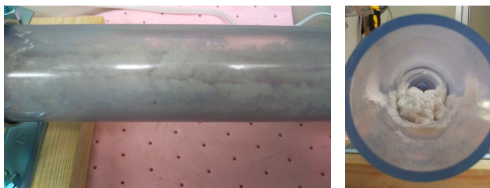
Figure 4. Clogging inside the sewer pipe on the 7th day in the simulated experiment (Observation point 4).
