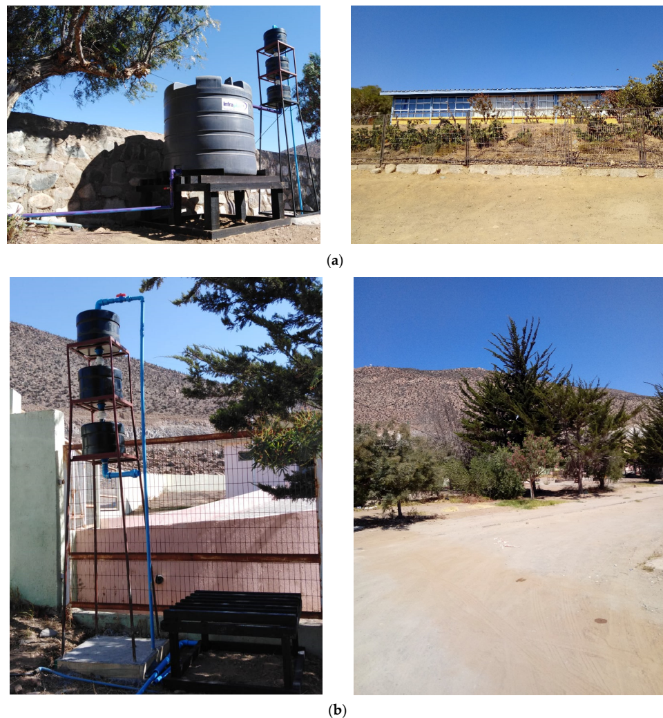
Figure 1. Greywater reuse system and irrigation area of Los Pozos (a) and José Santos Ossa school (b). The photographs on the right correspond to the area irrigated with treated greywater.
