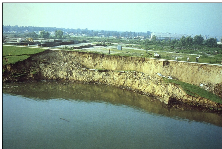
Figure 12. Bank failure of levee at Donaldsonville, Louisiana during the 1973 flood. Such failures are most common when water levels drop precipitously after prolonged high flows. Photo courtesy of J. David Rogers.
