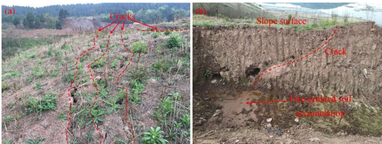
Figure 15. Characteristics of crack development before slope failure: (a) characteristics of slope surface cracks; (b) characteristics of section cracks.
