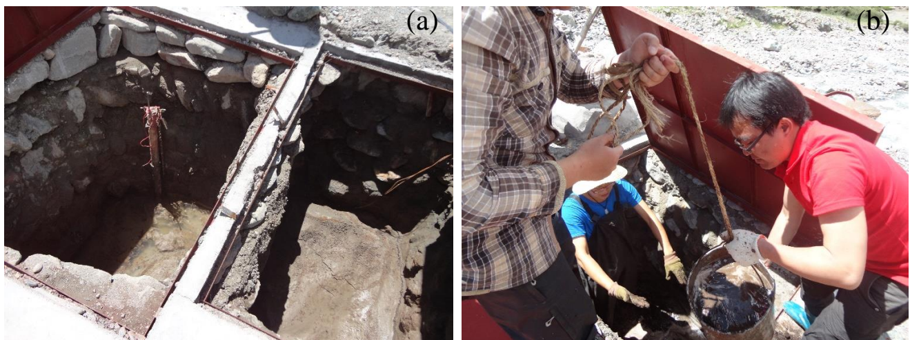
Figure 3. Two wells constructed of the hydrographic cross-section. (a) The silted-up wells. (b) Manual dredging from the water wells.
