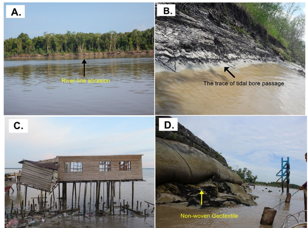
Figure 9. The impact of tidal bore propagation on the surrounding environmental conditions. River-line abrasion (A); coastal erosion at the edge of the river (B); local settlement destruction due to tidal bore (C); non-woven geotextile fabrics as coastal protection applied in several areas of interest (D).
