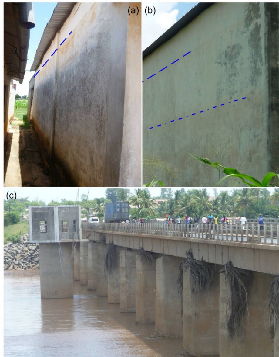
Figure 2. Field data evidence of January 2015 flooding event: palaeostage indicators for CP-01 (a) and CP-05 (b), where blue dashed lines show the water level (flood marks) at these points; Mocuba gauge station and bridge with palaeostage indicators (driftwood) (c).
