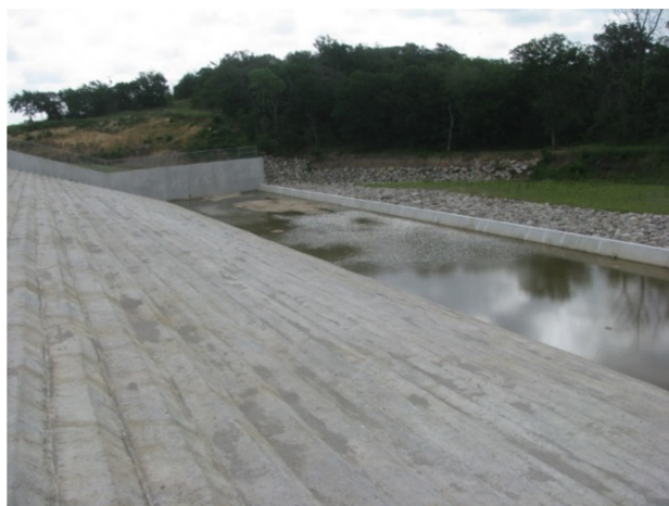
Figure 1. Constructed RCC beveled face stepped chute at Caney Coon Site 2 in Oklahoma (photo courtesy of USDA-NRCS).
