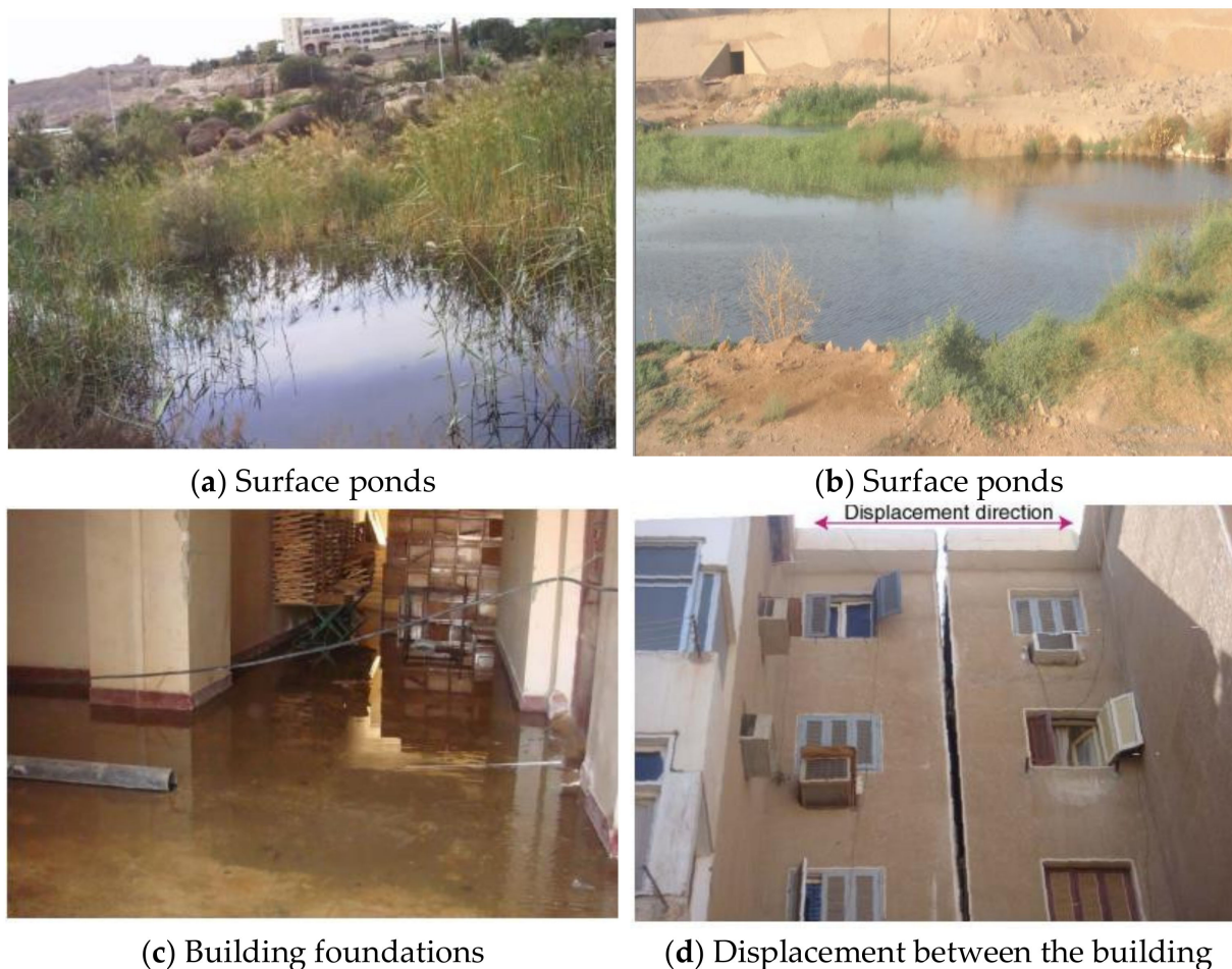
Figure 1. The effects of groundwater on the study area; (a,b) Formation surface ponds; (c) Flooding the foundations of buildings; (d) The appearance of displacement between buildings.
