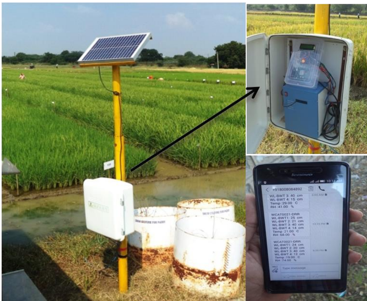
Figure 4. A smart irrigation device installed in the field.
