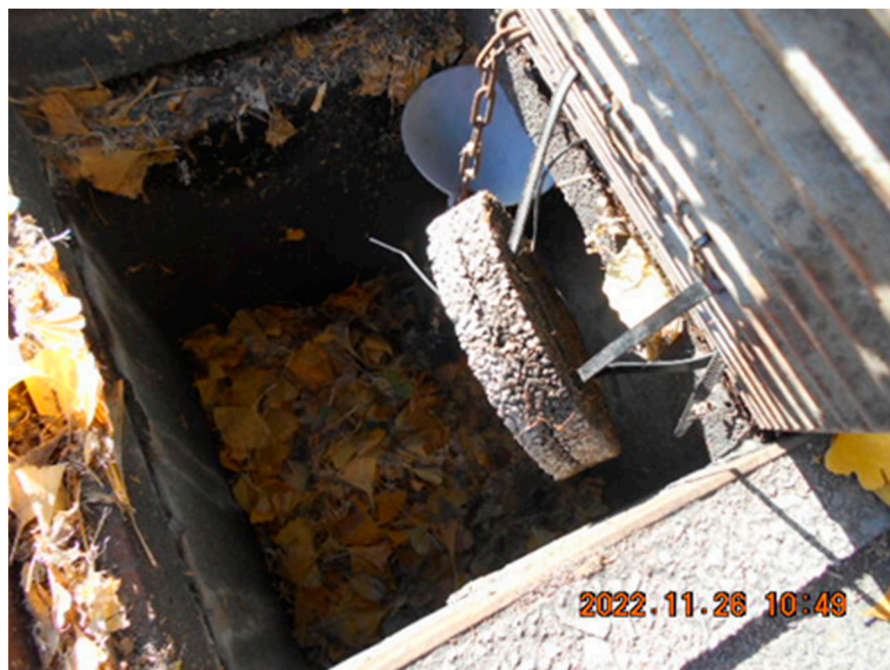
Figure 14. Hanging-type placement of the porous concrete at the same inlet as the one shown in Figure 1. The grating is open. Closing the grating results in the porous concrete board assuming a horizontal orientation.
