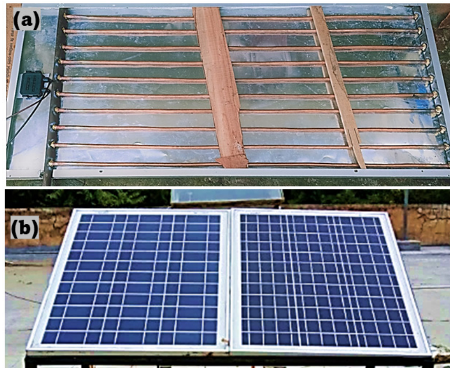
Figure 3. Installed experimental set-up.
