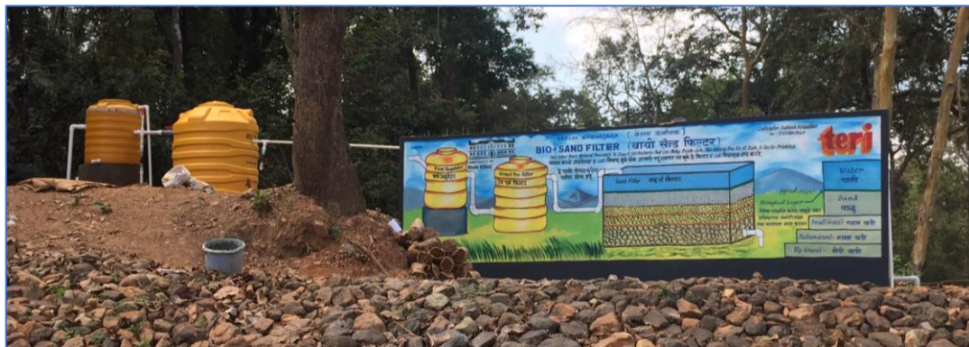
Figure 3. Picture of the IBF filter system. A diagram was painted on the filter wall giving a simple explanation of the system in both English and Marathi, the local language.
