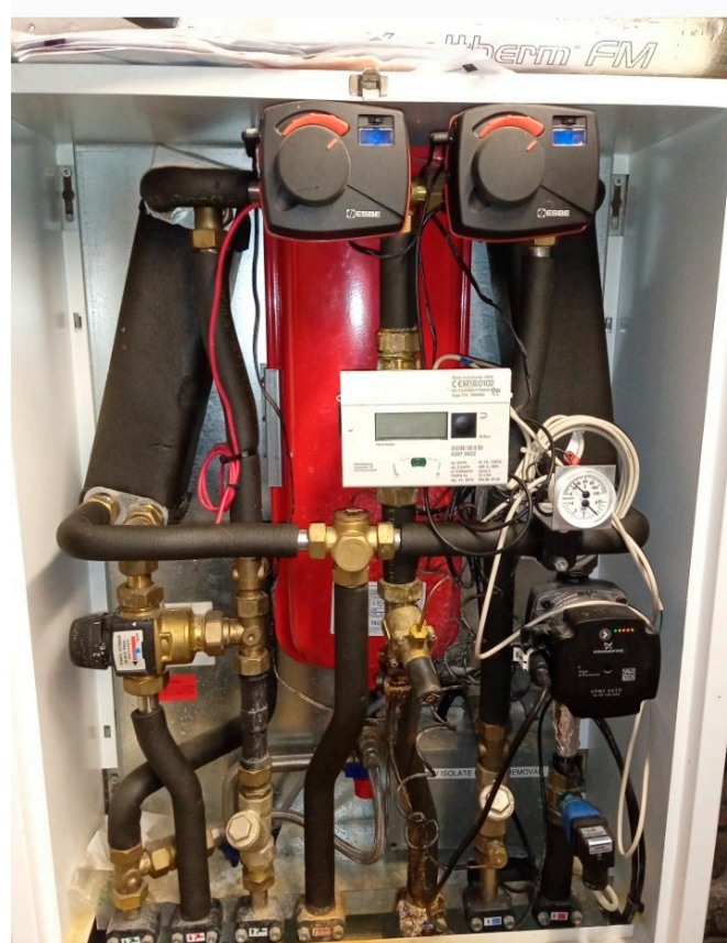
Figure A5. Heating interface unit of the pilot heat recovery system in the technical room.
