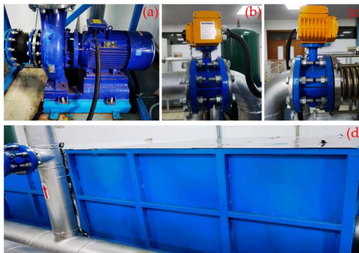
Figure 3. Physical pictures of the water supply module device: (a) QZHW200-250IA centrifugal pump; (b) motorized butterfly valve; (c) motorized regulating valve; (d) low-level water tank.
