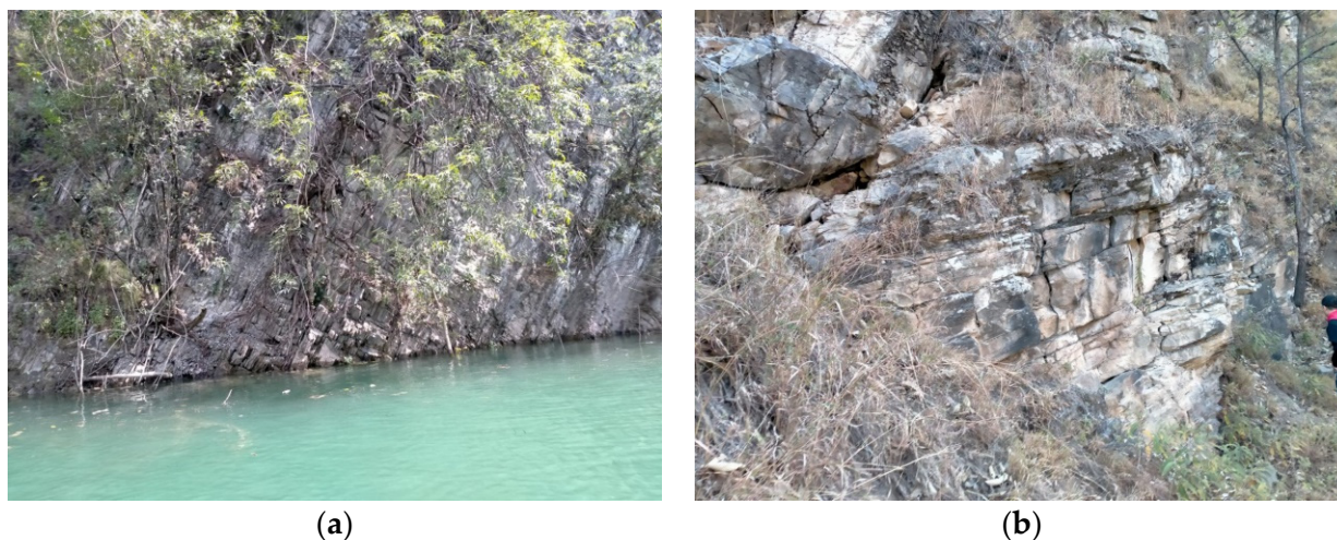
Figure 7. Toppling rock mass of the bank slope. (a) Near the reservoir surface at 1403 m; (b) at the elevation of 1540 m.
