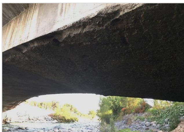
Figure 2. Erosion on the deck of the bridge.
