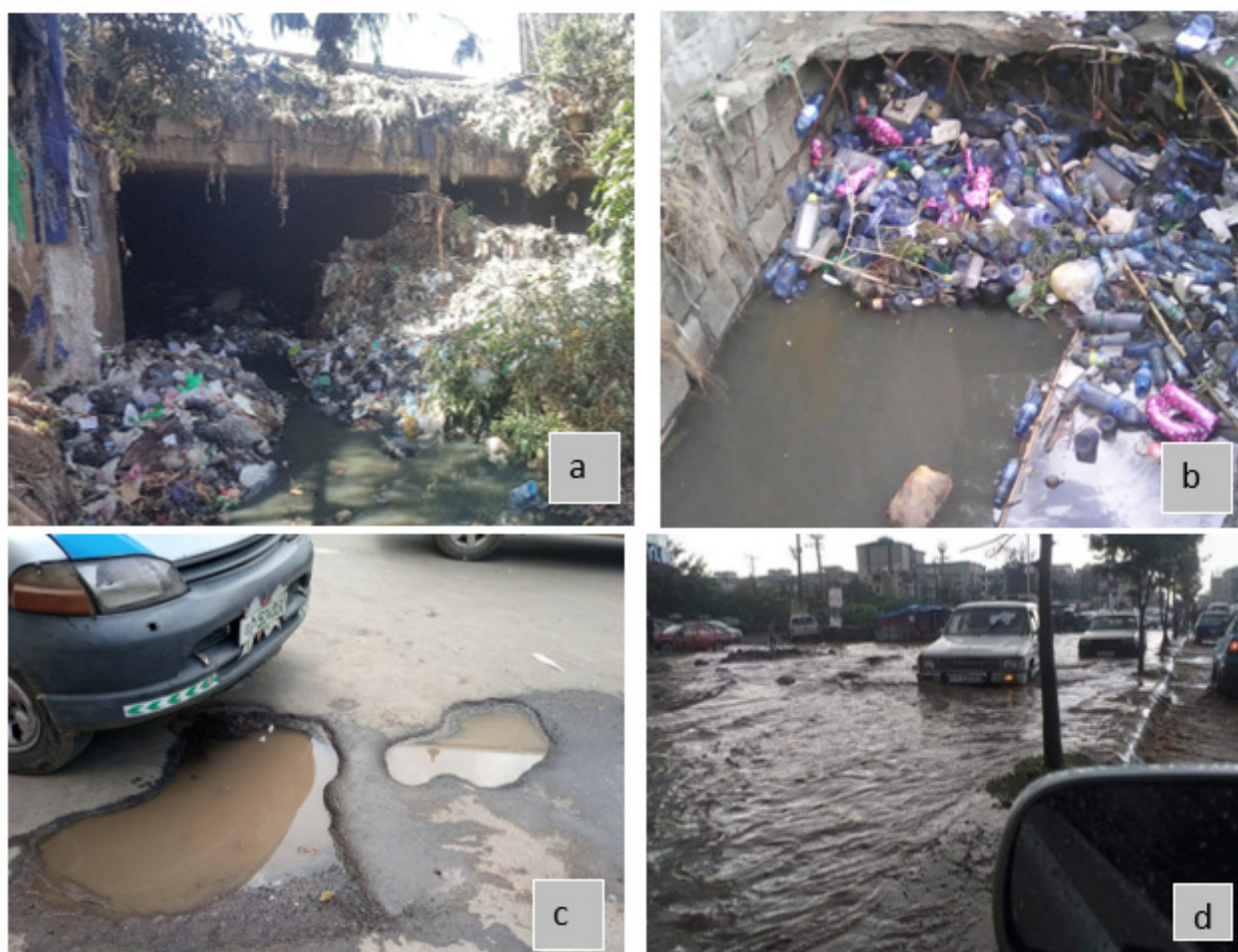
Figure 11. Solid wastes, dominant drainage failure causes (a,b), the impacts of poor drainage by creating potholes (c), and traffic disruption due to surface flooding (d).
