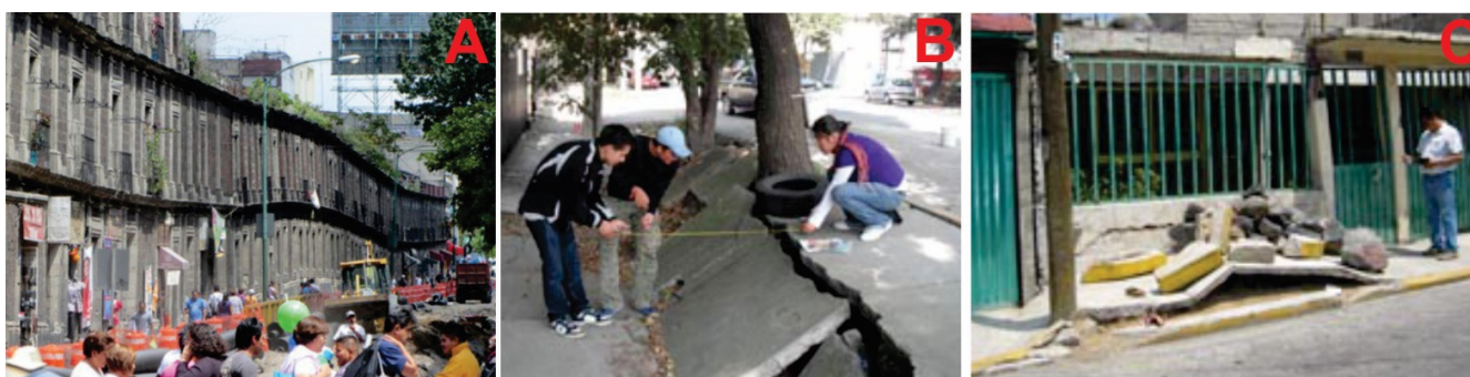
Figure 6. Damage due to land subsidence in Mexico City. (A) Vertical differential deformation [94]. (B,C) Damage to infrastructure [95].
