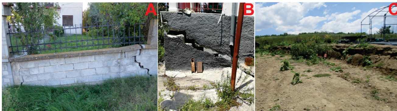
Figure 12. (A) Wall fence damaged due to vertical displacements of up to 30 cm at Valtонера village. (B) Damaged building wall and (C) greenhouse at Anargiroi village.
