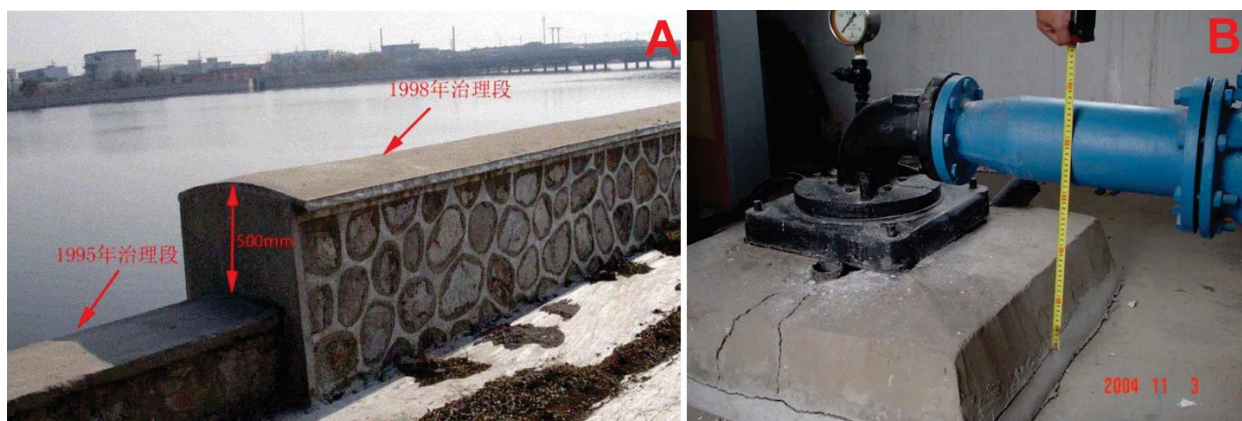
Figure 8. Land subsidence in the area of Tianjin city. (A) An increase in the height of the embankments due to land subsidence 1995 and 1998 1998 Governance Section. (B) Damage to the water supply system [156].
