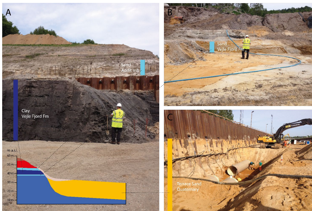
Figure 3. Post auditing the geological model on site. Sheet piling is visible in (A,C). Miocene sand from the Veje Fjord Fm (B) During construction, the groundwater table was lowered in several sections along the motorway with a suction cell system at the sheet piling, with suction cells every 1 m connected to larger pumps, picture (C).
