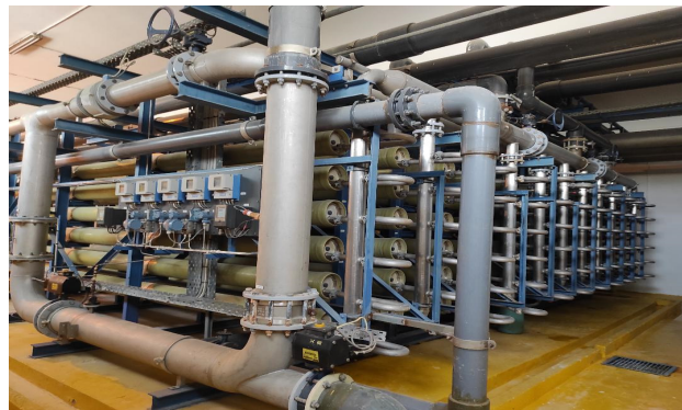
Figure 1. BWRO desalination plant.
