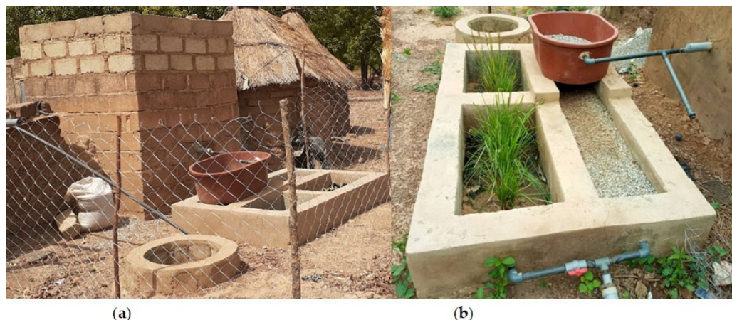
Figure 2. Complex shower room greywater treatment system planted with C. zizanioides under operation. (a) Beginning of study and (b) three months after operation began. Greywater flow and system components are shown on Figure 1.
