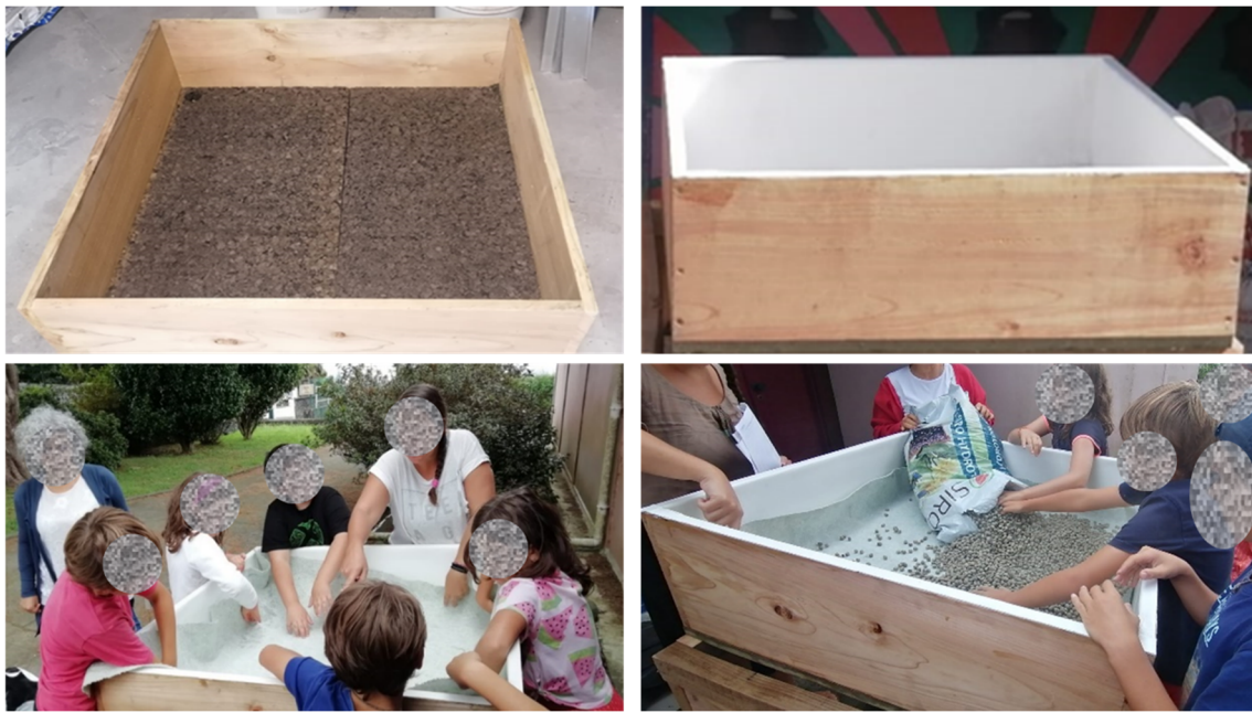
Figure 6. Installation of the expanded cork panels ( top left ), TPO membranes ( top right ), and the remaining layers ( bottom ).
