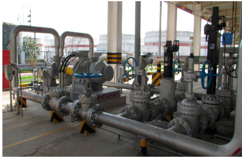
Figure 3. Experimental site of residual pressure power generation.
