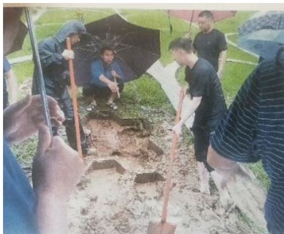
Figure 12. Insufficient downstream dam surface drainage.
