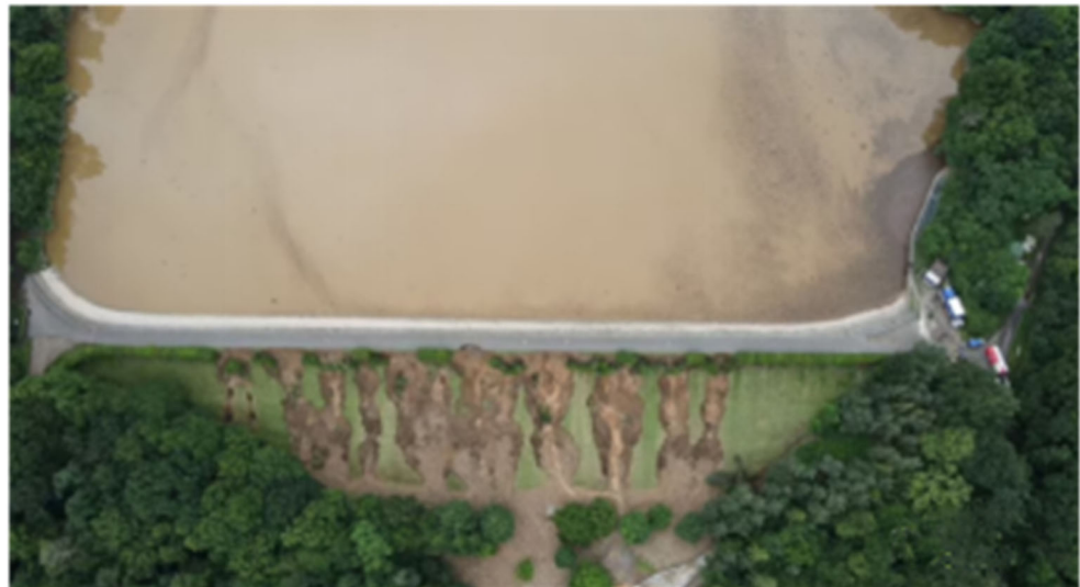
Figure 3. Scene of Steinbach Reservoir in Germany after overtopping.
