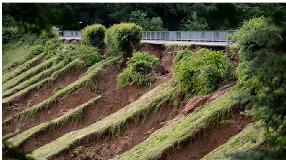
Figure 4. Downstream dam slope after overtopping of Steinbach Reservoir in Germany.
