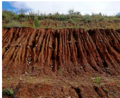
Figure 1. Erosion failure of heavily weathered granite slope.
