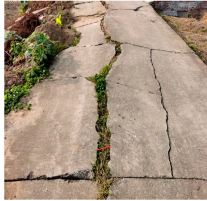
Figure 12. A damaged levee surface.
