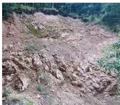
Figure 9. Fissures in rock slopes.
