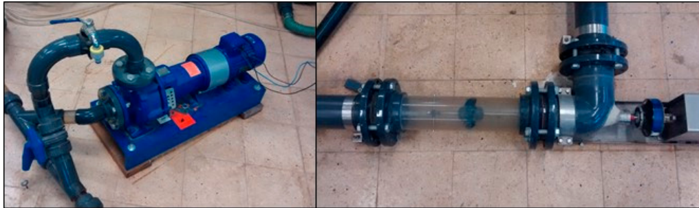
Figure 6. Hydraulic machines at IST-Universidade de Lisboa: PAT (left); and tubular propeller (right).
