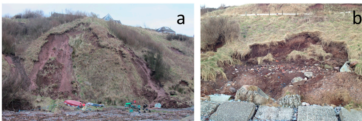
Figure 3. (a) typical translational slips; (b) typical deeper-seated slips on the study site.
