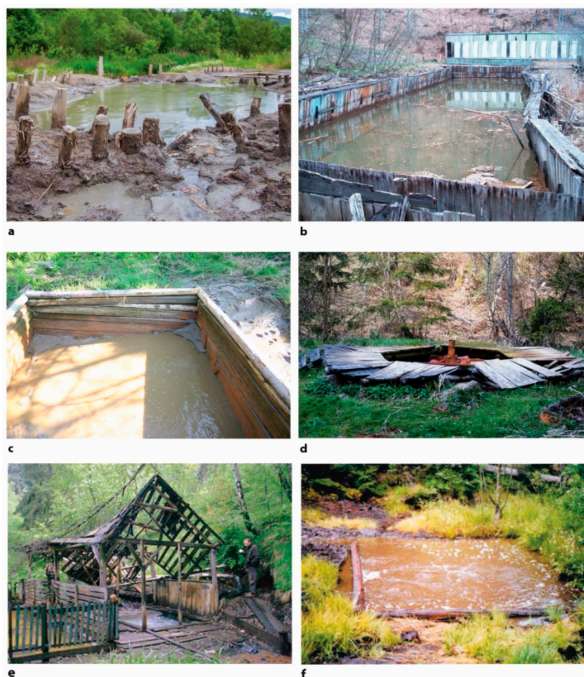
Figure 6. Ruined traditional baths in the 1990s: (a)—Parajdfürdő, (b,e)—Csiszárfürdő, (c)—Hammasfürdő, (d)—Szelterszfürdő, (f)—Vallató (source: Ars Topia Foundation).
