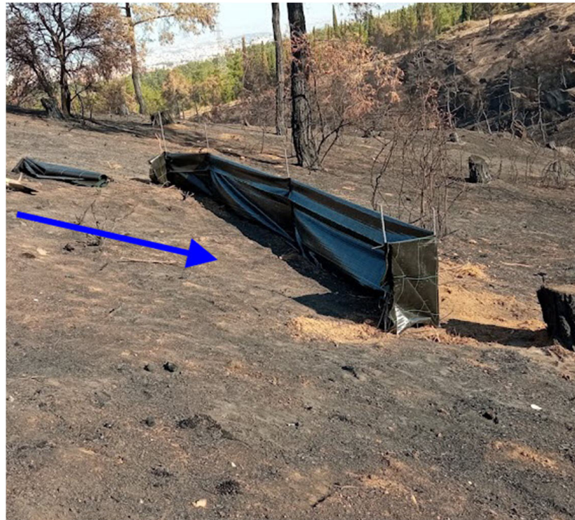
Figure 4. Silt fence installation process: the silt fence was fastened on 5 metal rebars. The blue arrow indicates the runoff direction.
