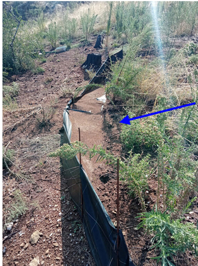
Figure 6. Silt fence operation: the silt fence has bended under the weight of sediment material. The blue arrow indicates the runoff direction.
