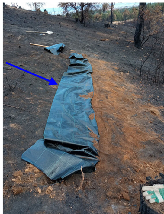
Figure 3. Silt fence installation process: the geotextile compacted with earth material in the trench. The blue arrow indicates the runoff direction.
