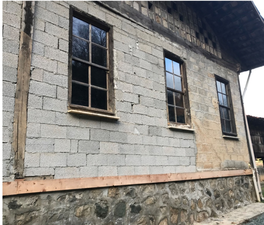
Figure 7. Site visit of a house in Çaglayan village in Fındıklı on 12th January in 2019. Maladaptation example of rebuilding the eradicated rear façade with briquette wall after the landslide in 2018. Source: Photograph by the first author.
