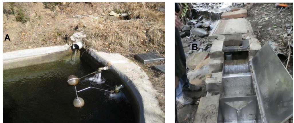
Figure 12. Installed mechanisms which regulate water extraction (A) and distribution boxes (B) restricting the amount of legally allowed water for exploitation.
