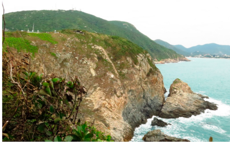
Figure 9. Collapsing observation post of Bokhara Battery between the two gun emplacements (with masks) (October 2017).
