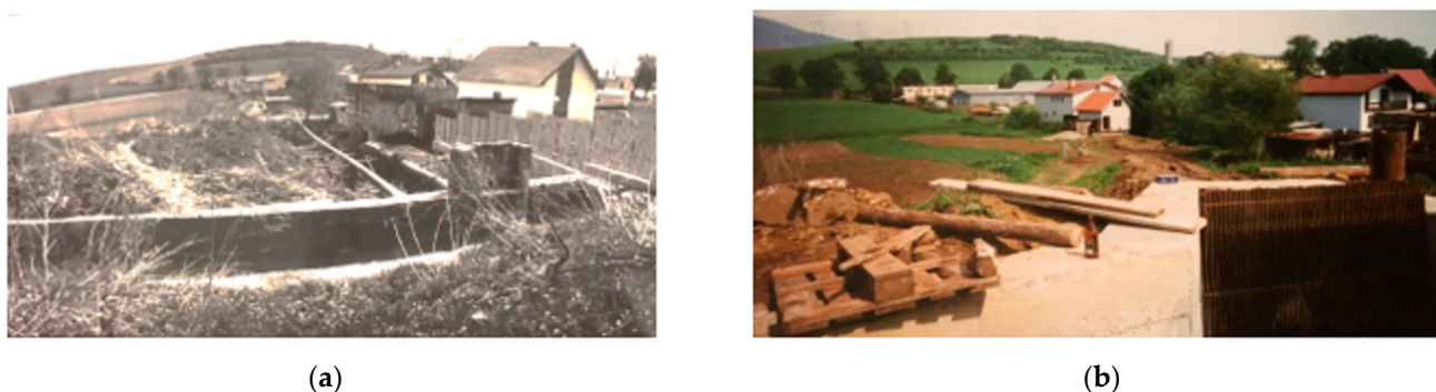
Figure 6. Process of the construction of SHP Žehrica and SHP Žehrica II. Source: Lukas Olejnik, accessed date: May 2019. (a) In the foreground the original entrance building, in the middle the remains of the mill, in the background the SHP building; (b) New entrance building of SHP Žehrica II., in the background the building of SHP Žehrica.
