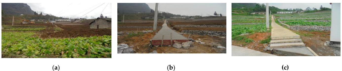
Figure 12. Land consolidation project in Bowangshan Town (hillside fields to terrace) (provided by Bowangshan Town): (a) before; (b) in progress; (c) after.
