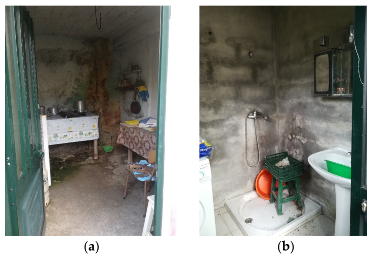
Figure 5. Building incompatible with residential use in the parish of Porto da Cruz: (a) interior space with humidity on the walls; (b) sanitary installation with several infiltration and humidity problems.
