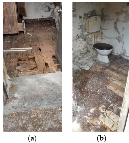
Figure 6. Building not suitable for residential use in the parish of Santo António da Serra: (a) ground floor with rotten wooden flooring; (b) sanitary installation with several infiltration and humidity problems.
