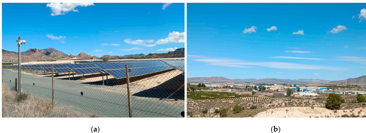
Figure 15. Photovoltaic plant (a); industrial estate (b) in the Ricote Valley Region. Source: Own elaboration, authors.
