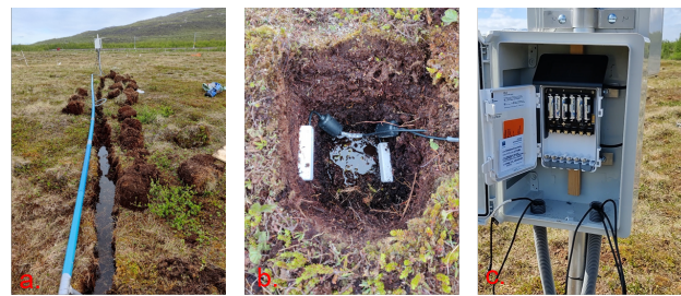
Figure A1. Fieldphotos of the volumetric water content sensor installation: (a) Main trench dug to install PVC pipes that contain the sensor cables. (b) Sensors installed at the depths of 0.1 m and 0.25 m in the soil profile SP1. (c) ZL6 data logger and housing box connected to the sensors.
